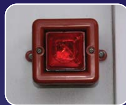
External panic alarm / beacon
