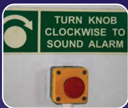
Internal panic alarm
